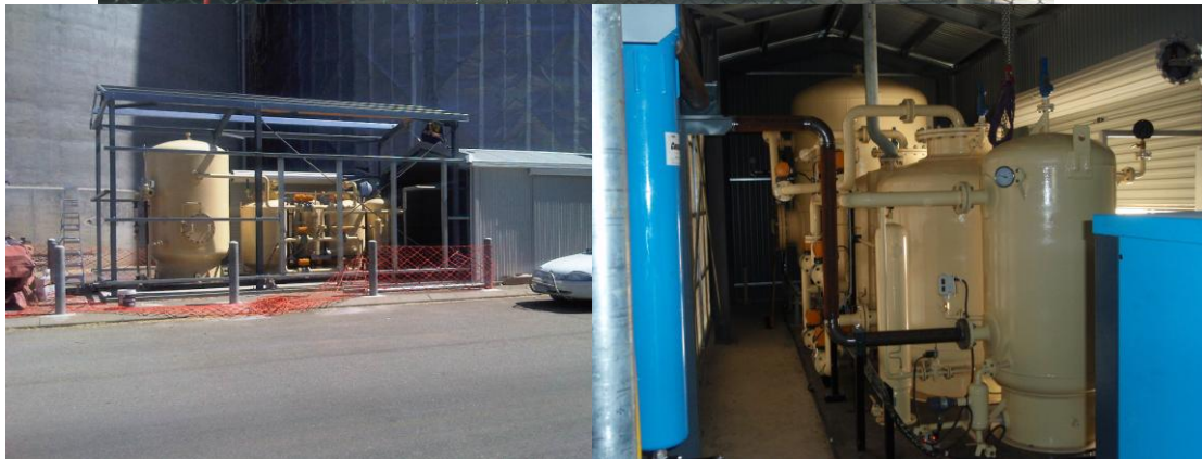
Figure 3. A 350 m 3 /hour PSA nitrogen generator has been installed at the CBH Albany grain export terminal (35°1'50.90"S 117°53'10.54"E). The generator is plumbed to a bank of 10 x 10,000 tonne concrete cells.
